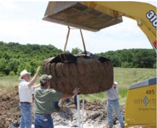
Install pipes in the ground before placing tires, leaving an extra length of inlet pipe that can be cut later to the desired height.
